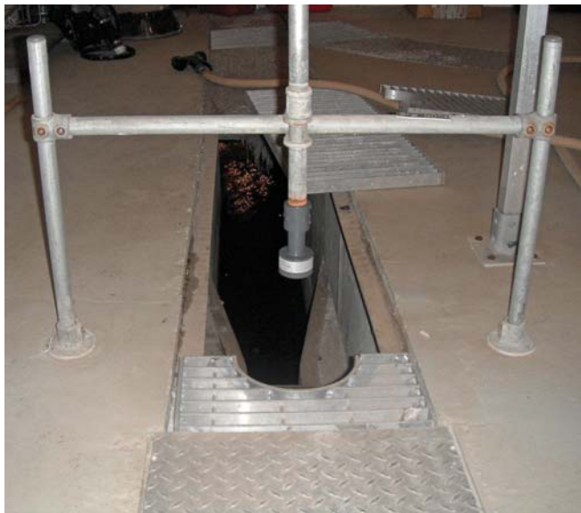
Intrinsically Safe Ultrasonic Sensor Installed above a Parshall Flume
