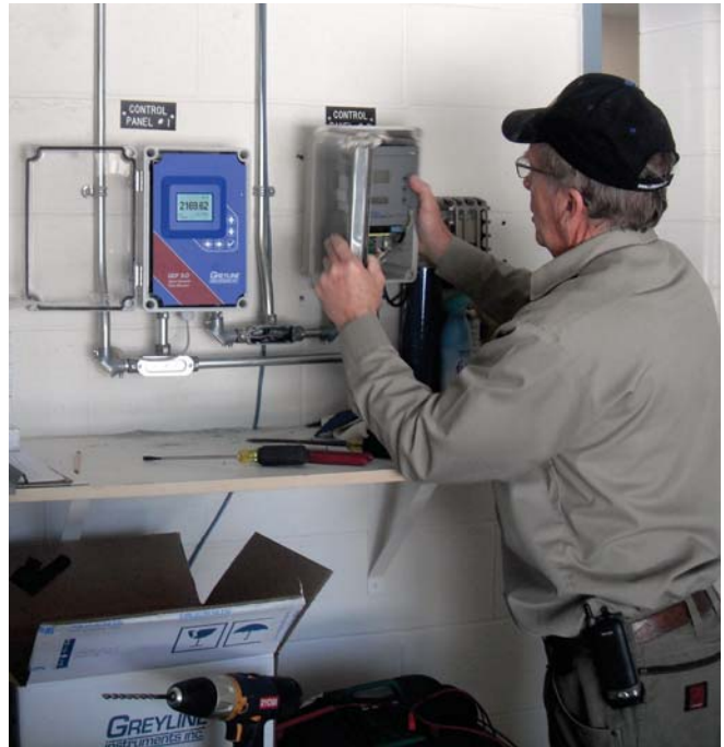
Contractor Bob Crawford of Marleau Mechanical Installs OCF 5.0 Open Channel Flow Monitors
